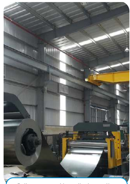
Coil corrugated iron discharge line
