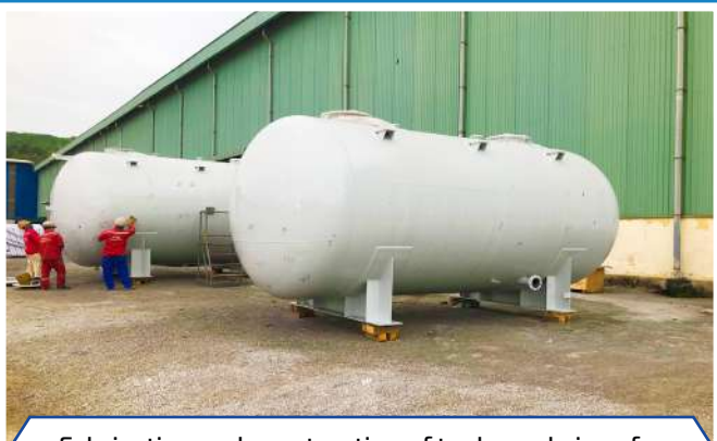
Fabrication and construction of tanks and pipes for Nghi Son 2 Thermal Power Plant
