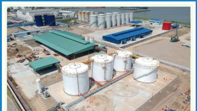
EPC Fuel Depot Project - Topsolvents Client at Dinh Vu Industrial Park, Hai Phong
