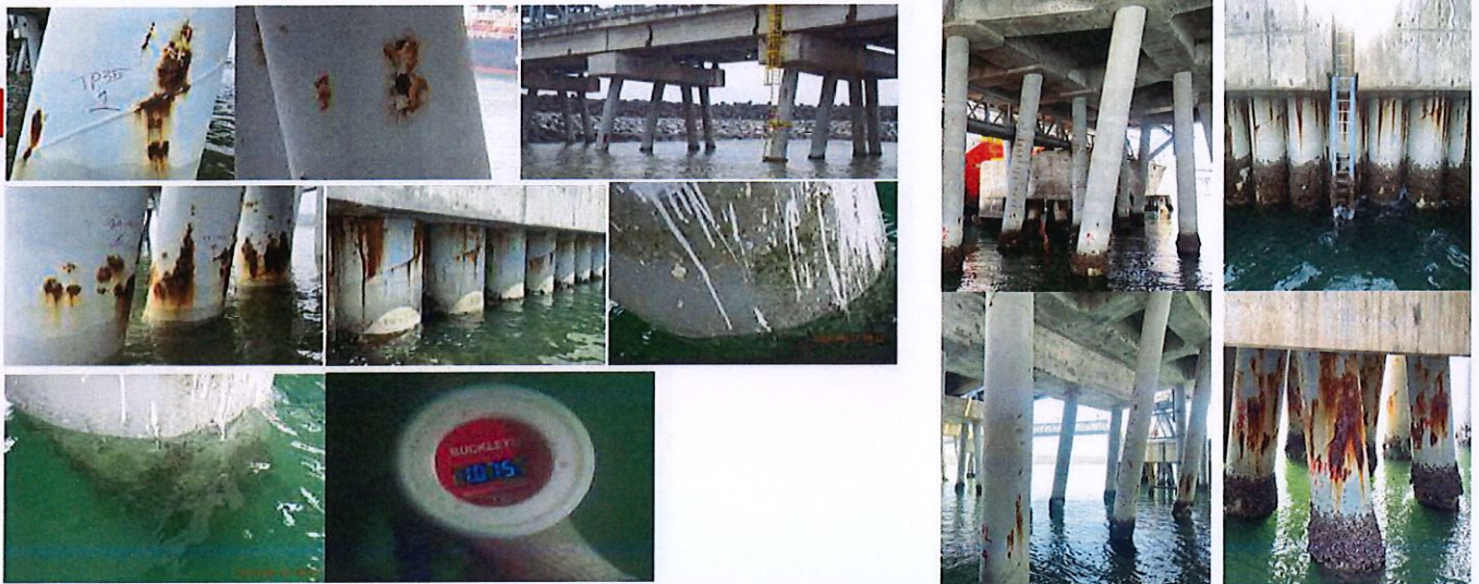
Figure 3. Atmospheric Zone, Splash Zone Pile Corrosion and Marine Growth.
